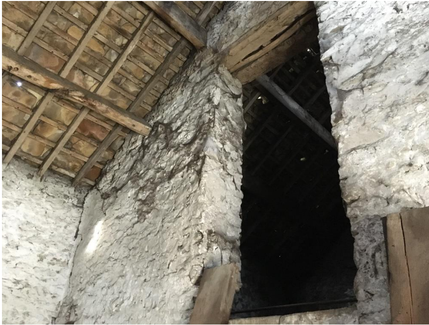
Fig.14: roof to through passage, and access doorway to the north loft from the passage
