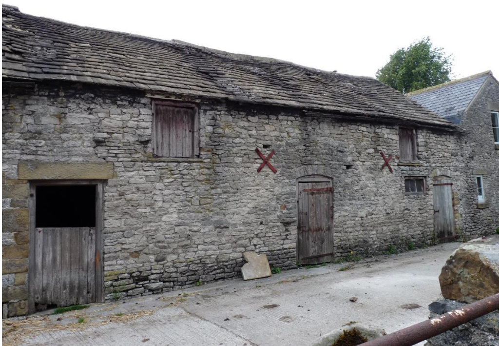
Fig.8: cowhouse in north part of the range, from the east, with central passage doorway
