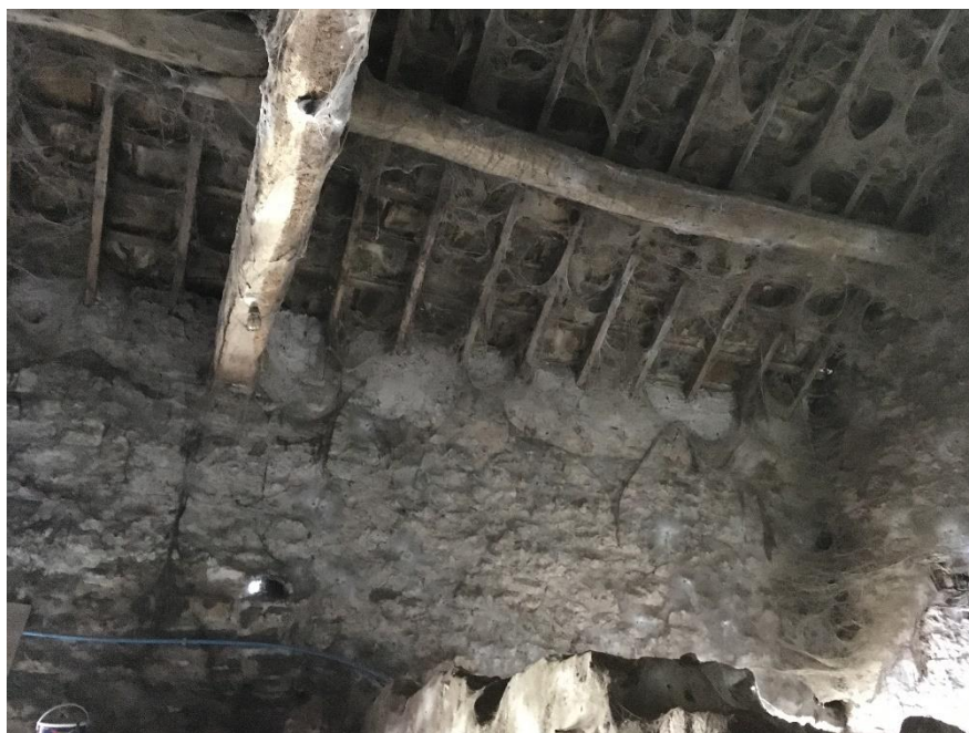
Fig.15: south bays with partial cross wall and roof truss, from the east
