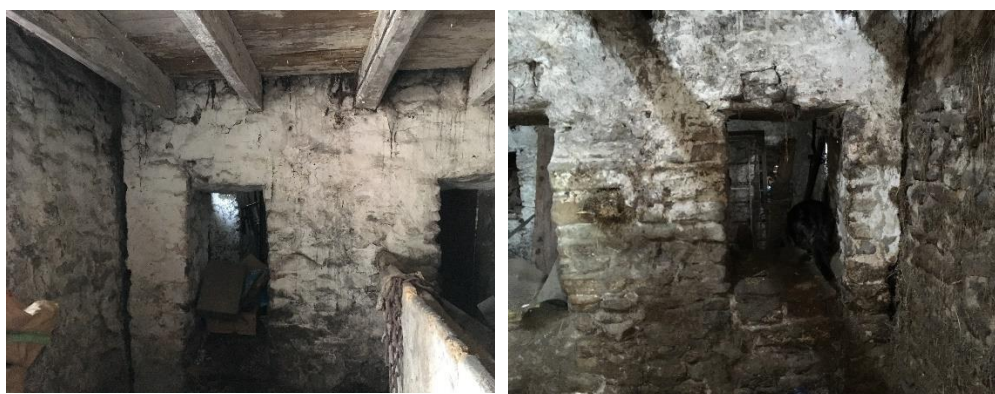
Fig.30: proposed doorway locations in unit 1 (north wall LH and south wall RH)
