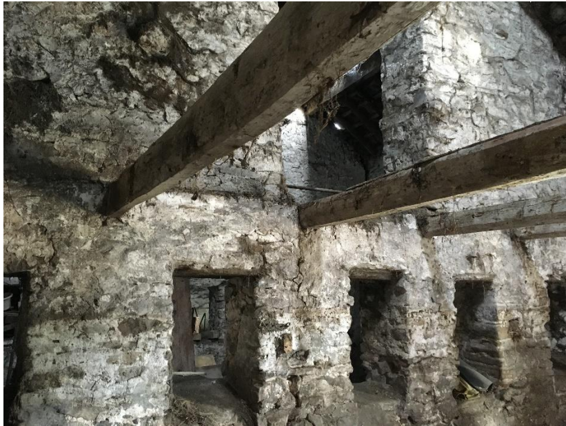
Fig.12: feed holes and loft floor joists in the south cow house, from the SW.
