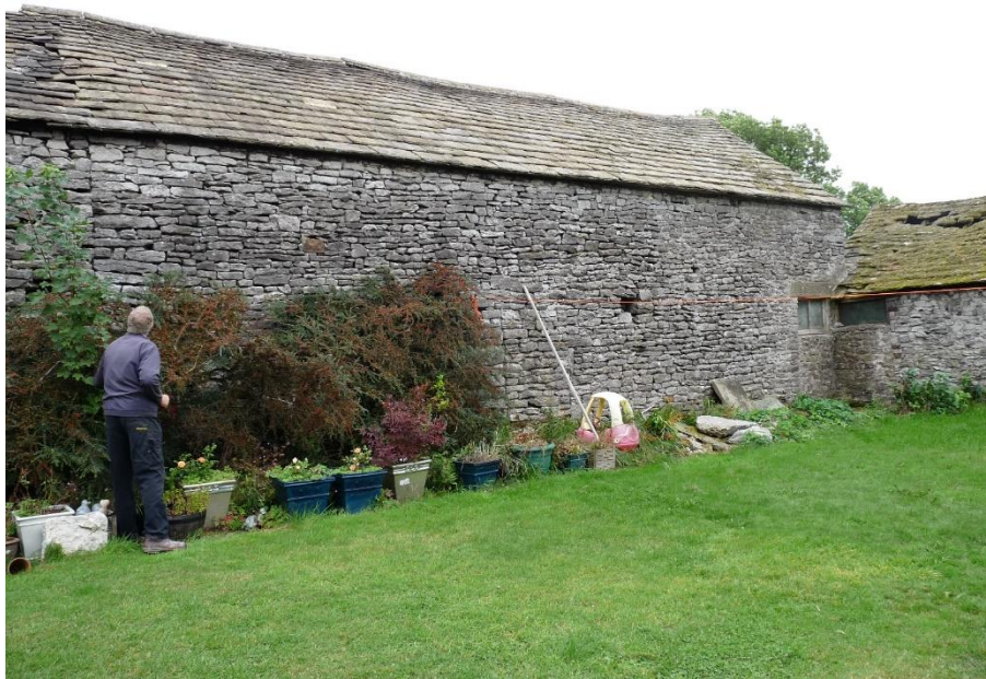
Fig.6: west elevation of south part of linear range, with straight joint visible to left
