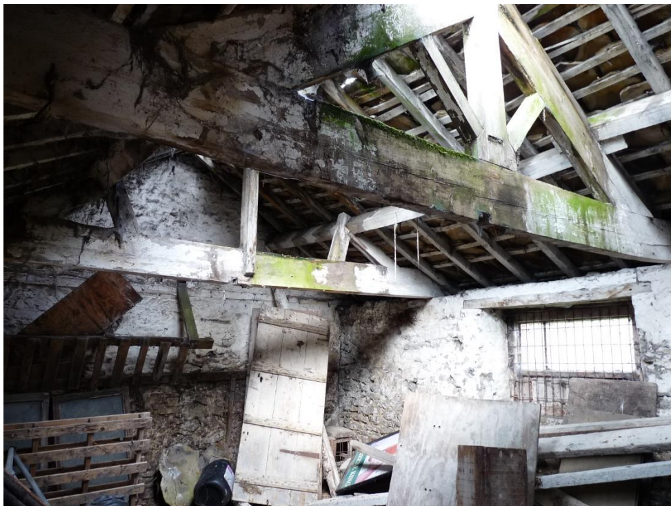
Fig.21: west cow house interior from the south-east, with inserted partial truss to left
