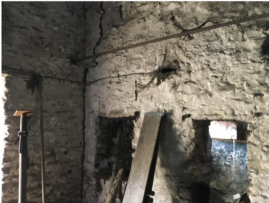
Fig.11: south side wall to passage, with feed openings and tie-rod, from the NW
