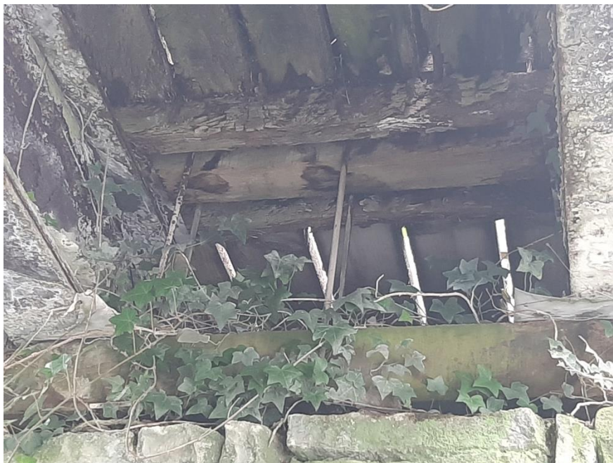
View at top of Pier showing deterioration of timber
