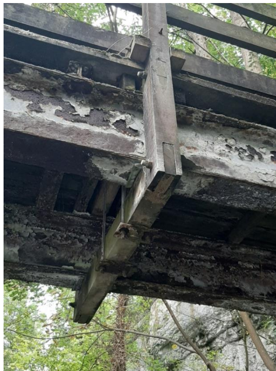
Underside of bridge – flaking paintwork/ exposed steel
