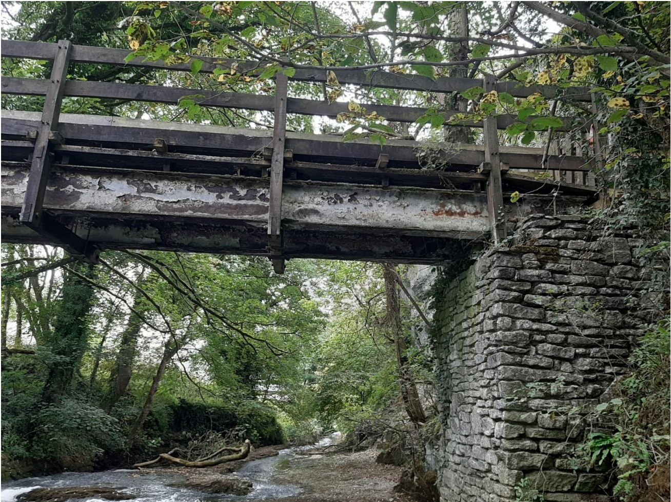
View looking towards the Western Abutment – flaking paintwork on steel
