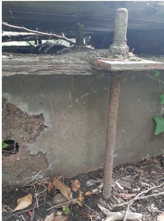
End of southern beam on Western Abutment – delamination of steel (top flange)
