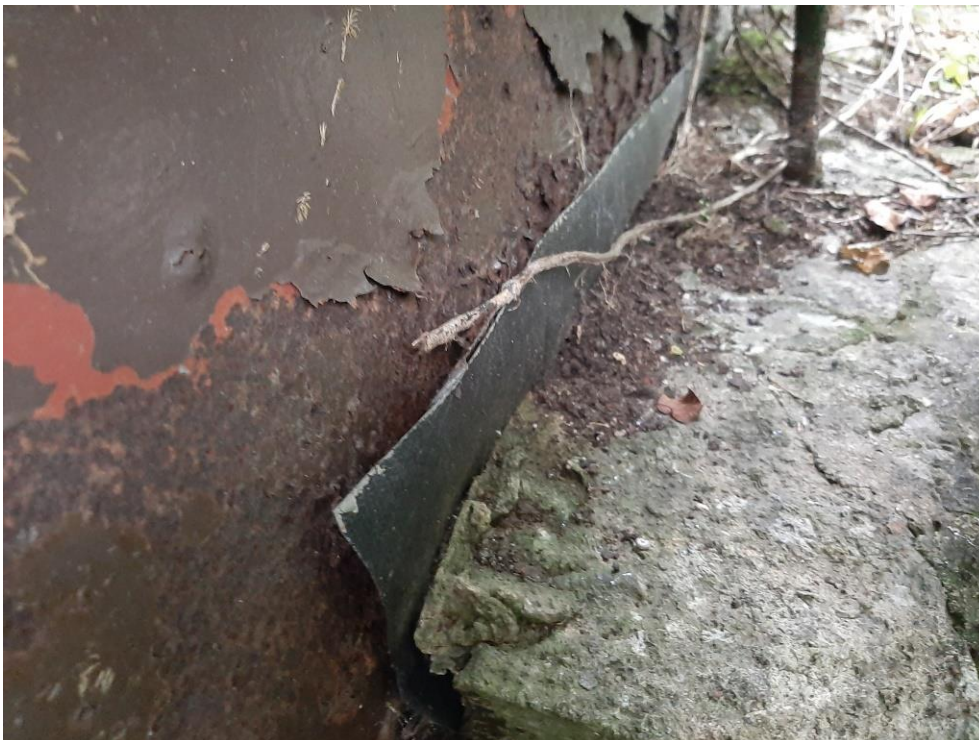
Steel sat on pier – flaking paintwork/ exposed steel
