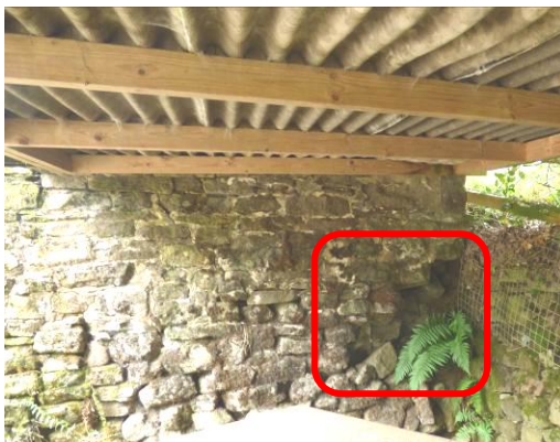
Photograph 17. Area of wall collapse of B2c.
