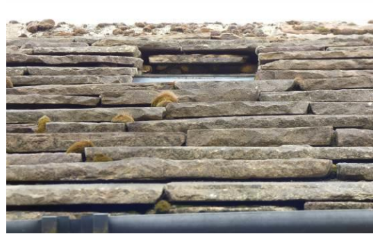
Photograph 2. Example gaps beneath roof tiles and adjacent to the skylights on the front elevation.
