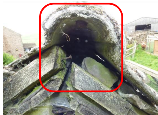
Photograph 12. B2a, location of cavity at roof peak
