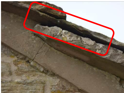
Photograph 5. Example gaps beneath roof tiles on the north-eastern gable.
